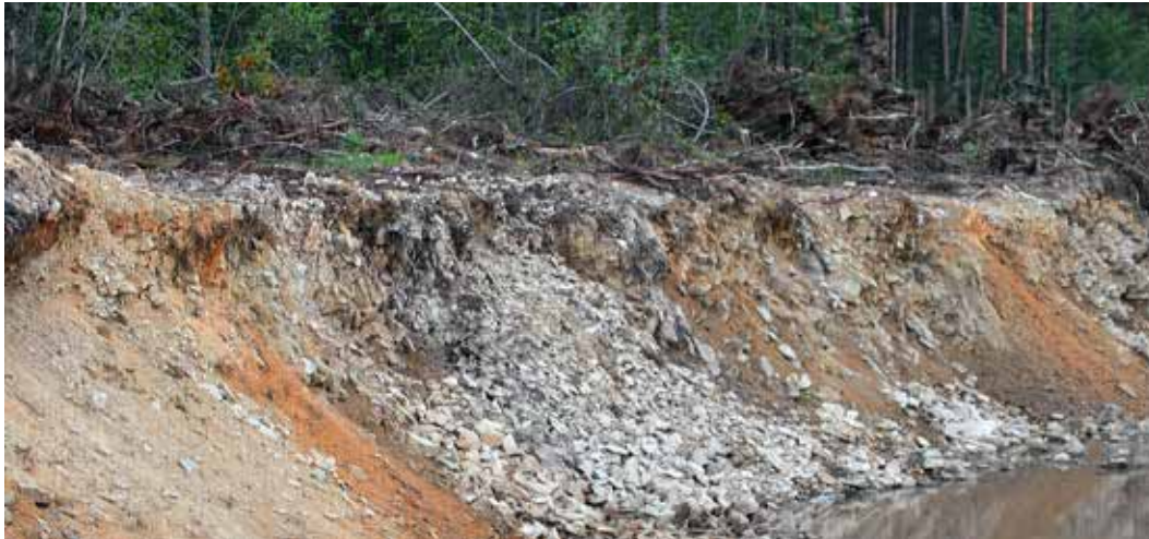
Fig. 1. Surficial residuum and talus exposed by a bulldozer on the foundation pit wall of a garage cooperative project, southern City of Neryungri. Horizontal scale: 1 cm–0.75 m. Photo by the author
